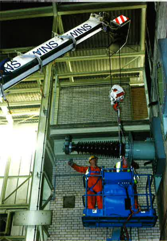
A 132,000 volt porcelain insulator is carefully removed during dismantlement works to make way for new cutting-edge switchgear at EDF Energy's St John's Wood substation
